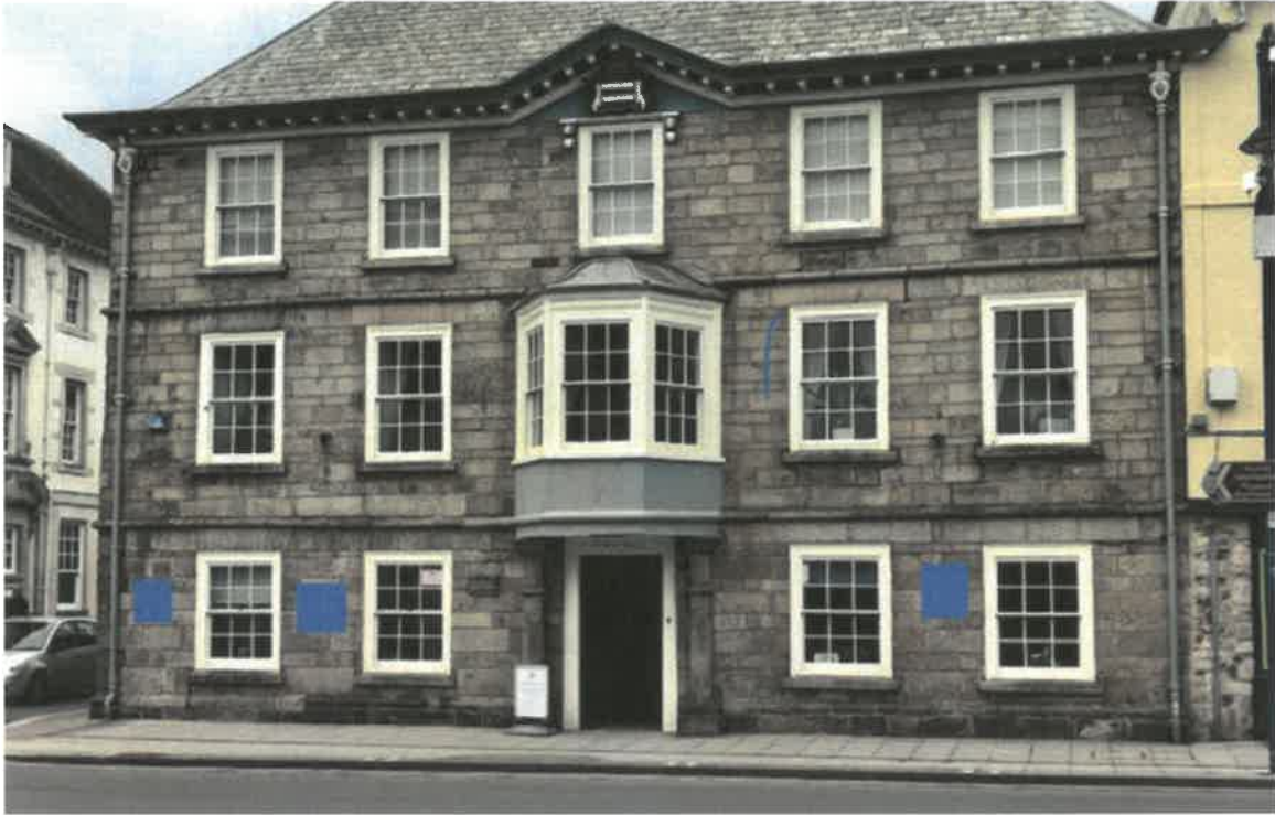
Option 1. The Town Hall. This is our preferred location due to its central location and visibility. The blue squares represent three possible fixings.
