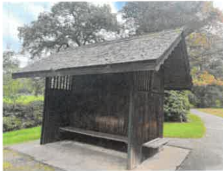
Some tiles on the rotary club shelter roof may need attention (sorry, no close up images)
